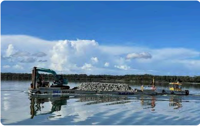
Project contractors are moving reef material for the intertidal Sydney Rock Oyster Reef Restoration project in Port Stephens, New South Wales. Image: M&J Marine.
